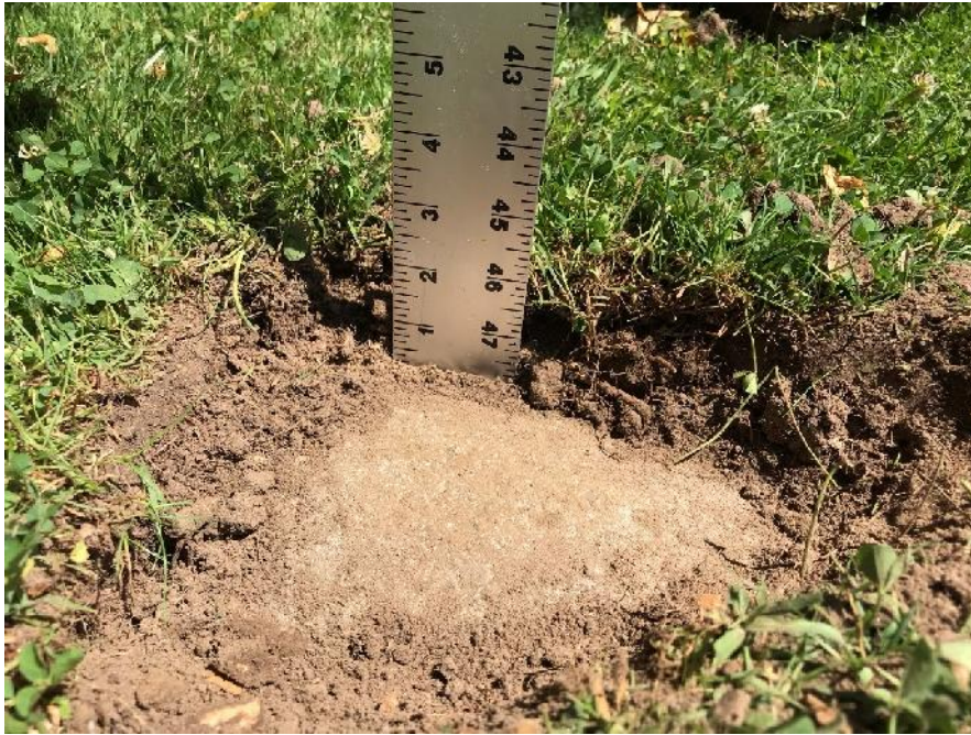
Figure 7: Depth of piped watercourse <3”
